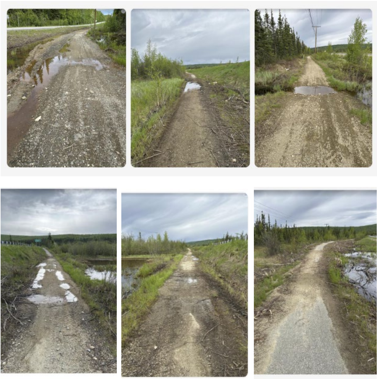
Ballaine Path images showing flooding of the path and signs of recent flooding
